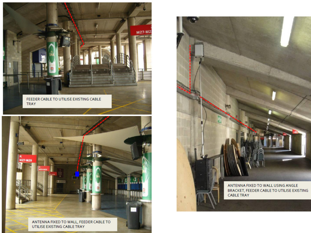
Figure 3-10: Example of cable routes inside a stadium (Twickenham Stadium)
