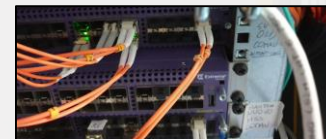
Switch connected to HSS
