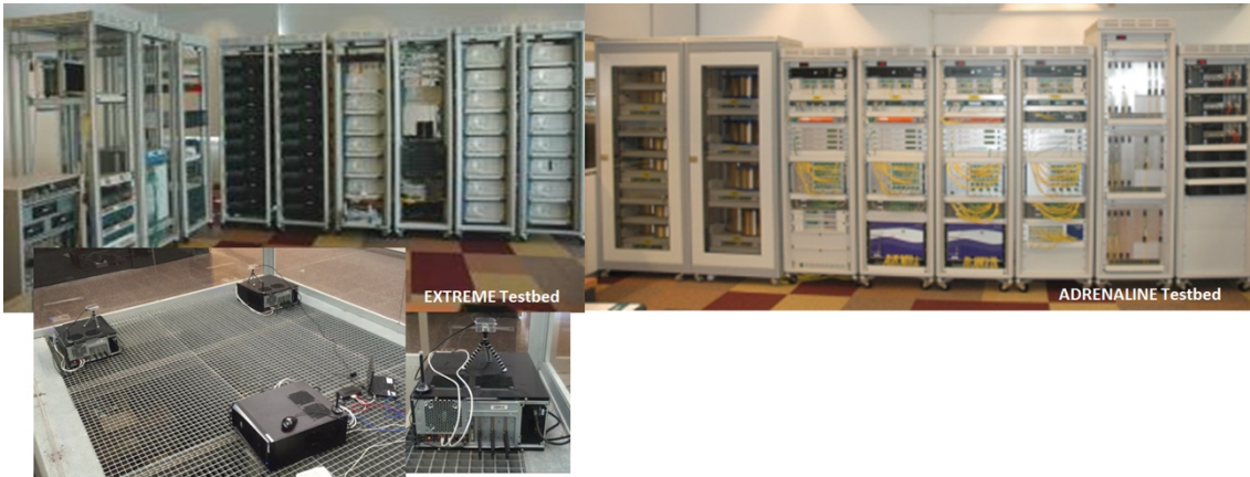
Figure 2: Exemplary equipment used for demonstration 3
